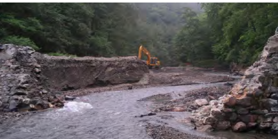
Demolition of the Mendaraz dam in Urumea River (Gipuzkoa). BIDUR transboundary cooperation project for the management of Urumea and Bidasoa Rivers. Gipuzkoa Council (IKT), Government of Navarra (GAVRN) and General Council of Atlantic Pyrenees.
