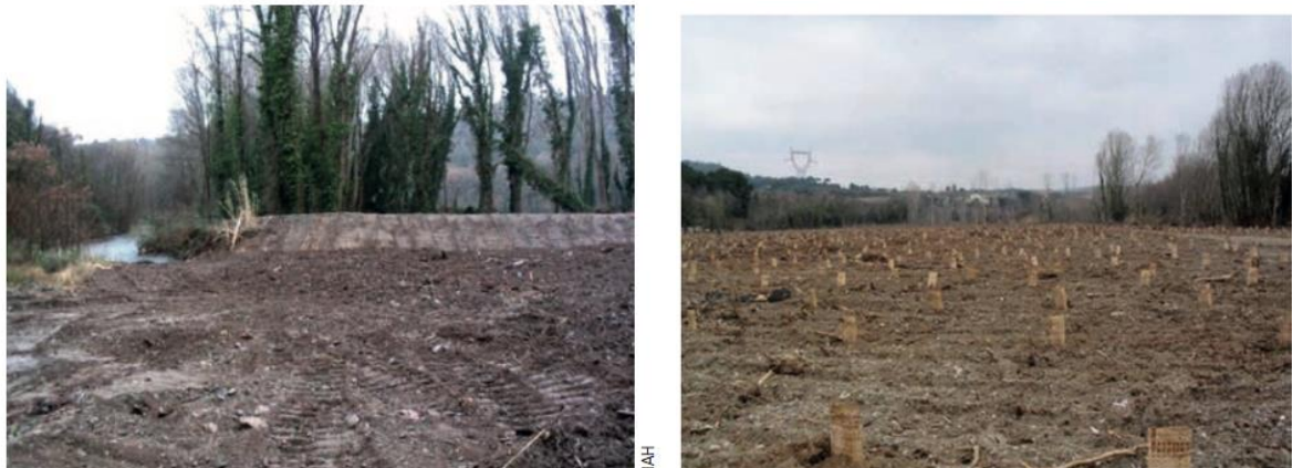
Figure 9. On the left, the newly constructed levee delineates the area. On the right, 5000 trees are planted in the area to decrease flow velocity during floods. Source: Syndicat intercommunal d'aménagement hydraulique des bassins de la Clamoux, de l'Orbiel et du Trapel (SBCOT)
