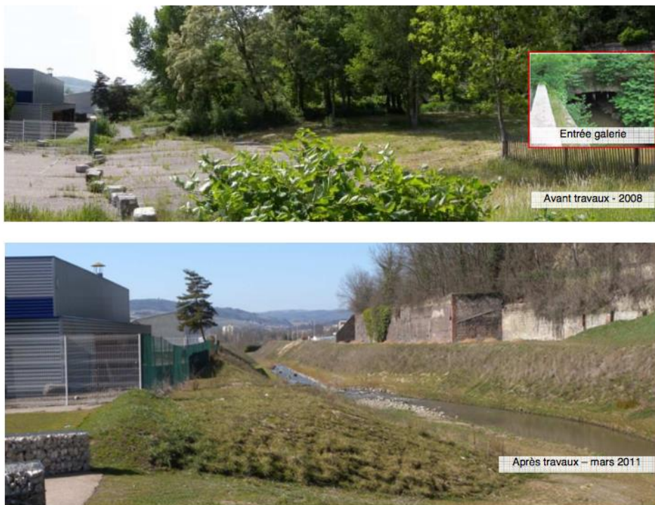
Figure 21. A view of the deculverting works: on top, the situation prior interventions; below, the reopened channel is pictured in 2011. Source: Saint'Etienne metropole.
