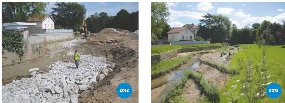
Figure 24. A section of the works completed on the Yzeron, at Charbonnières-les-Bains. Source: Sagyrc, Syndicat intercommunal du bassin de l'Yzeron.
