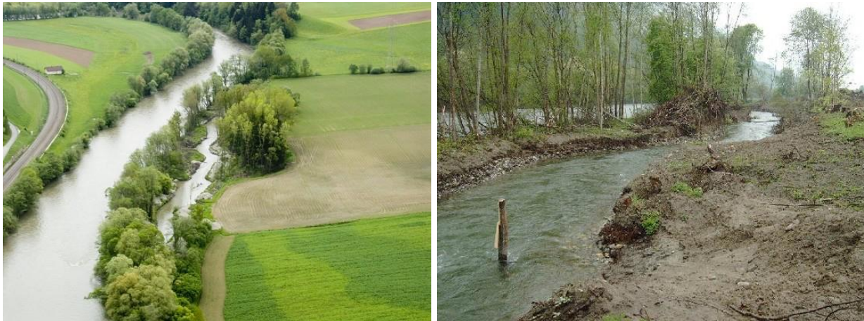
Figure 13. An abandoned channel is reshaped, and reconnected to the main channel at Thalheim. Source: Laymans report on “LIFE-UPPER MUR mur[er]leben 2003-2016”.
