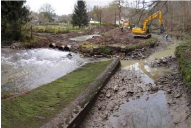
Figure 1. Works for weir removal at Spontin (source: LIFE project «Walphy» Layman's report).
