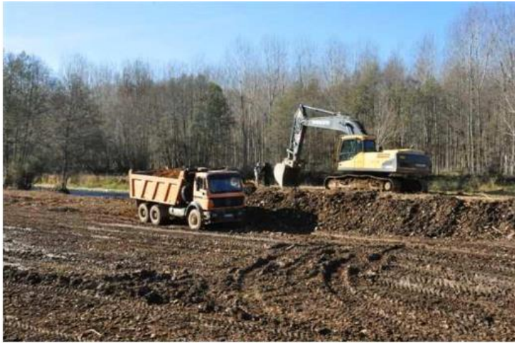
Figure 7. An artificial levee is lowered to recover lateral connectivity (source: Duero River Basin Authority – Confederación Hidrográfica del Duero).
