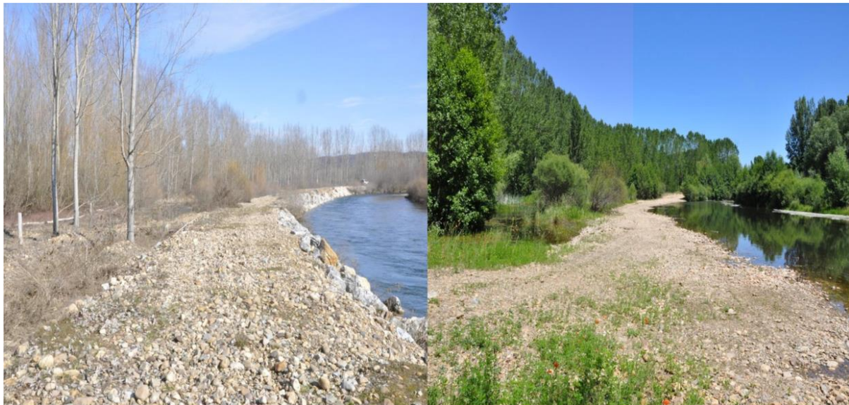
Figure 8. River bank protections were also removed along the river: on the left, the situation before the project; on the right, the river is reconnected to its floodplain (source: Duero River Basin Authority – Confederación Hidrográfica del Duero).
