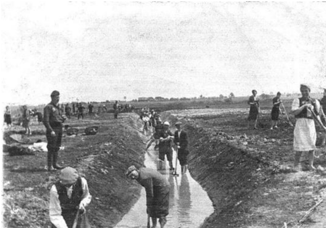
Figure 13: Drainage works in Krowie Bagno by prisoners of the German-Nazi forced labour camp in Krychów.
