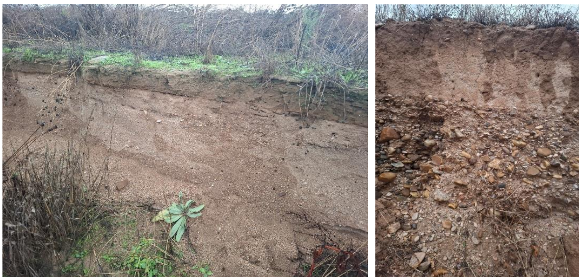
Figure 46: Alluvial deposits forming an aquifer layer (left), Conglomerate layers of sand and stone are vulnerable to erosion (right).
