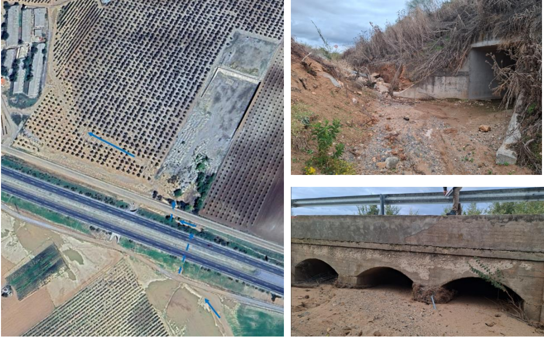
Figure 29: Ramabujas stream flows through a culvert under the highway (left) and bumps into the embankment of the secondary road (top right), where it flows 30 meters west through 3 small culverts to continue its way downstream (bottom right).
