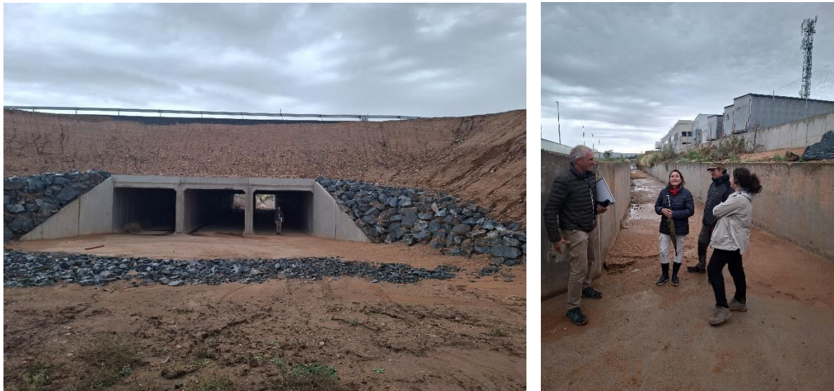
Figure 52: The new culvert construction under the TO-23 highway, with three passages, each having a flow area of 10 m 2 . Downstream of the culvert, the canal has a flow area approximately half of the culvert's capacity.
