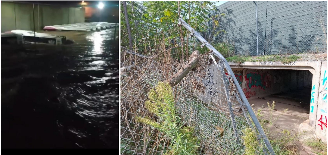
Figure 55: During DANA the Toledo bus terminal close to the Ramabujas was flooded (Left). Suntory, at more than 1 kilometre distance from the Ramabujas, was flooded as well. The culvert construction under the railway near Suntory was unable to process the flood water. The branch of a tree hanging in the fence indicate the water level during the flood (Right).
