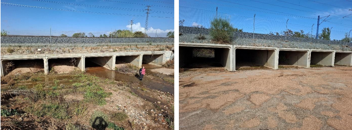
Figure 53: Two large culvert constructions under the railroad, each has five passages with a flow area of 5m 2 .
