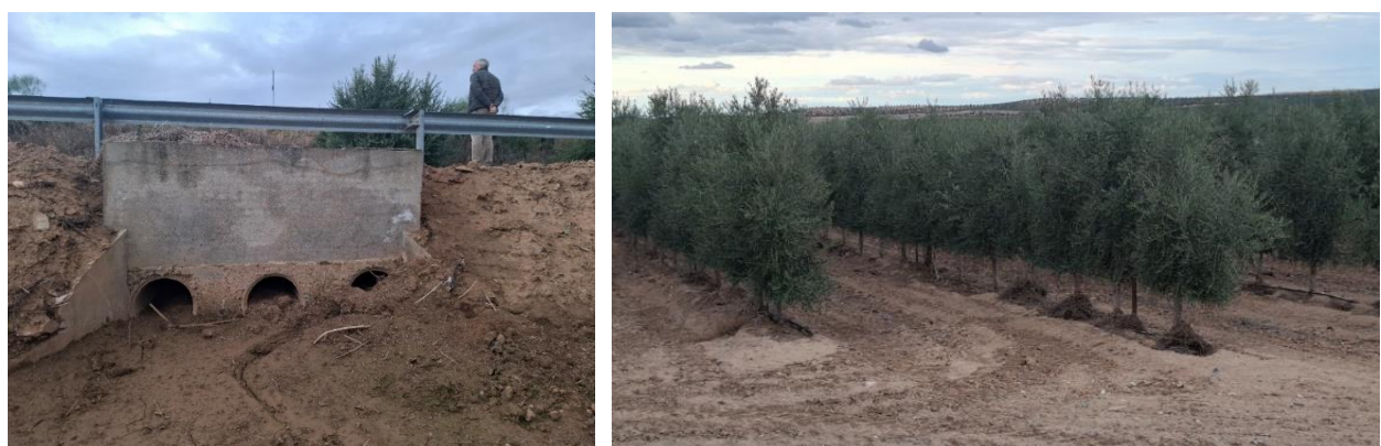
Figure 34: The smaller culvert under the secondary road couldn't handle the amount of water. The road flooded and water continued its way downstream through the olive field. Flood marks can be seen at the trunk of the trees.
