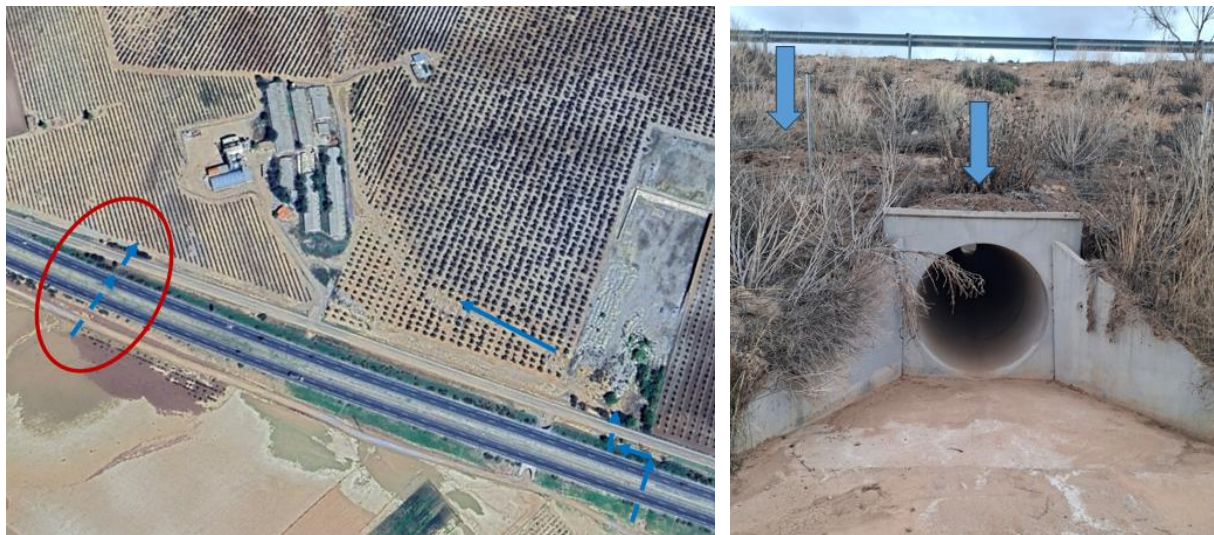
Figure 33: Flood marks under the highway revealed high water levels (3 meter) at the upstream side of the highway.
