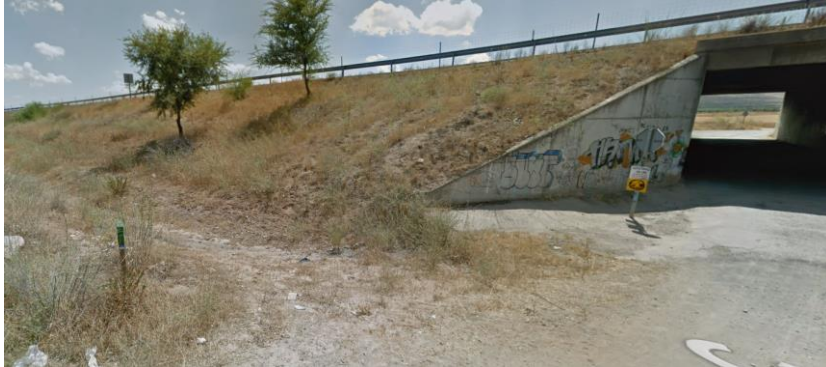
Figure 65: The start of the canal with a 90 degrees angle between the incoming water (through the tunnel) and the canal. In case of DANA much of the water will flow straight into the village instead of flowing into the canal.
