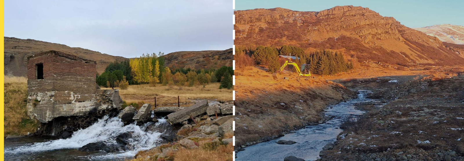
Figure 6. The Ytri-Hraundalur hydropower dam site at Melsá River in Iceland, (left) before and (right) after the removal works © (left) Jóhannes Guðbrandsson, and (right) Iðunn Hauksdóttir
