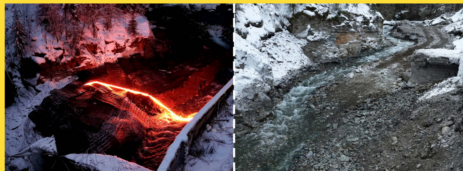
Figure 8. (left) Detonation of explosives during the removal of a dam on the Vinstra River, Norway, and (right) restored site after the dam removal © Kjetil Rolseth
