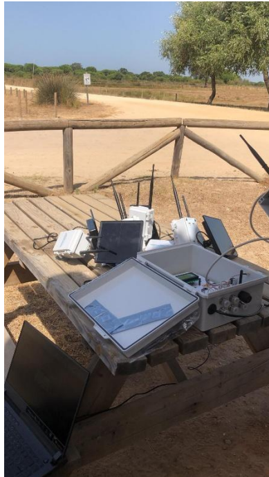
Picture 9. Image of the tests conducted in Doñana, where the system was assembled and powered on for the first time.
