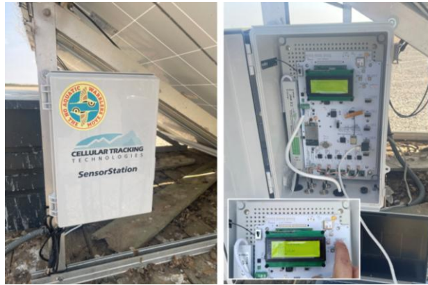
Picture 2. Photograph of the CTT SensorStation installed in Boada in August 2025. The system is powered by solar energy generated by the solar panels owned by FGN.
